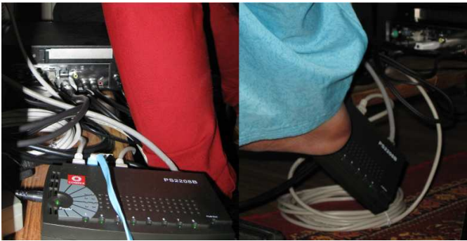
Figure 5: State of cabling at Radio Bundelkhand. The device in the front in both the images is the Ethernet switch connecting the two GRINS computers. The device seen in the background is the Linux computer of GRINS.
